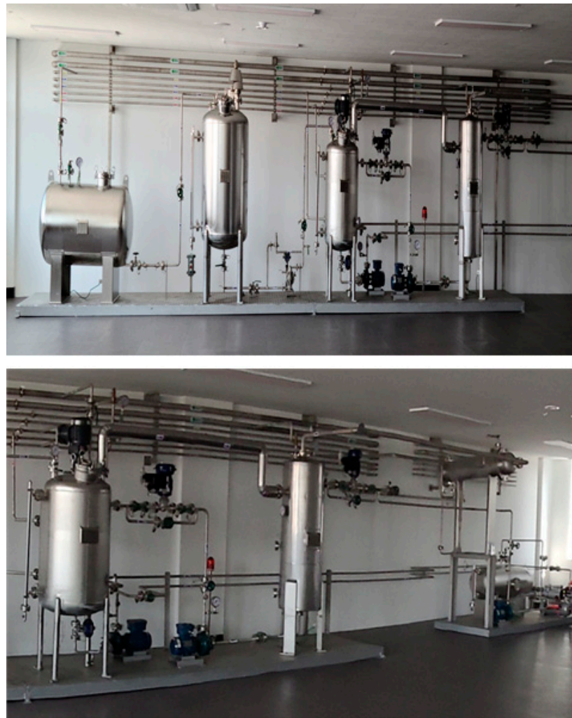
Figure 7. A photograph of the installed pilot plant.
