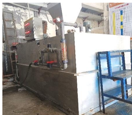
Figure 4. The flocculant addition equipment.
