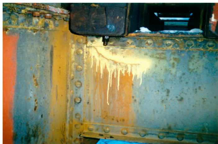
Figure 1. Illustrative picture of a fatigue crack occurrence in the web of the stringer.
