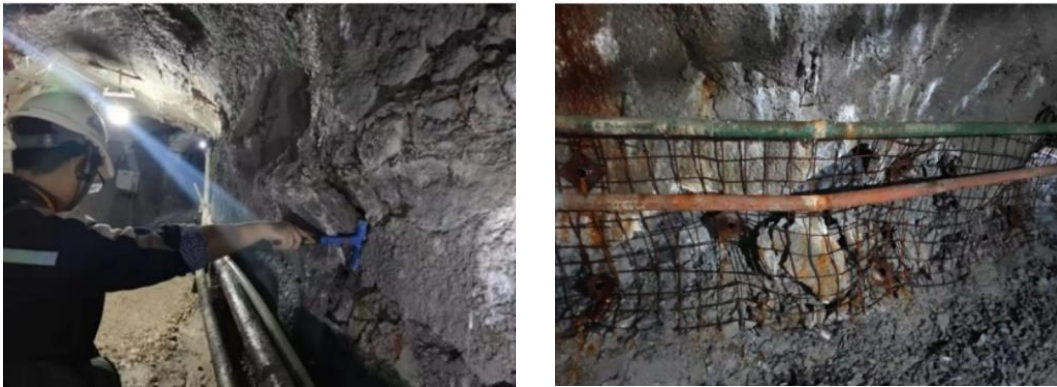
Figure 9. Deformation damage of quasi-ramp support in I-8# orebody.
