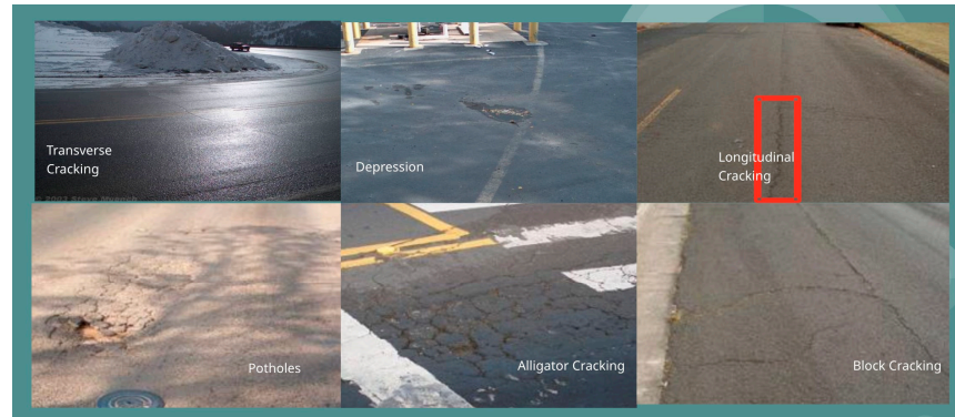
Figure 1. Types of pavement distress.
