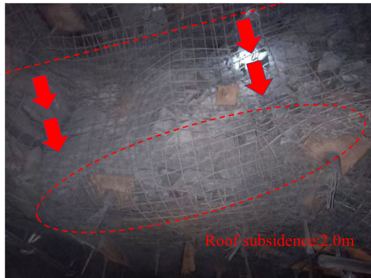
Figure 4. Subsidence of Roadway Roof.
