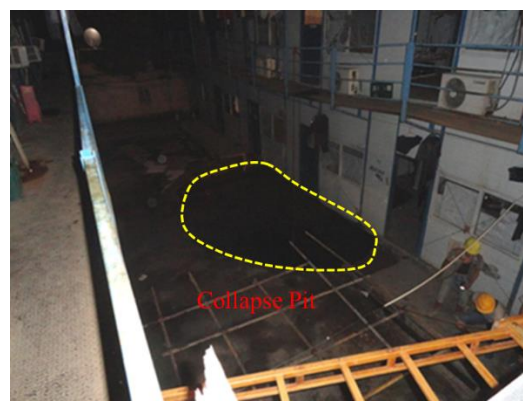
Figure 4. Collapse pit on Parrot Avenue in Wuhan, China.
