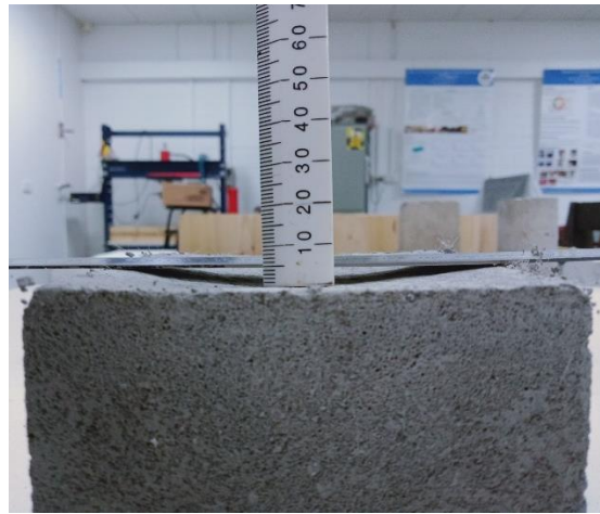
Figure 4. Unstable void network for low-density foam concrete.
