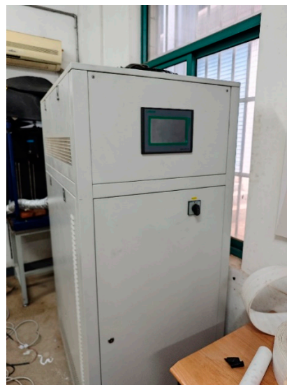
(a) Circulating pump control panel
