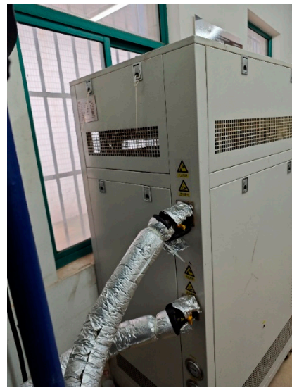
(b) Circulating pump liquid inlet and outlet
