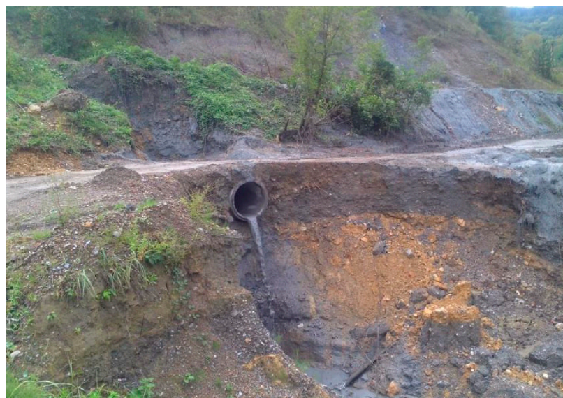
Figure 5. The damaged pipe culvert on the western field. Reproduced with permission from the Water Institute “Jaroslav Černi” [10].
