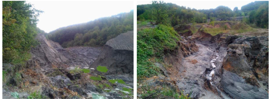
Figure 4. The damaged embankment of the eastern field. Reproduced with permission from the Water Institute “Jaroslav Černi” [10].
