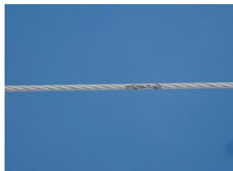
Figure 1. Phase-to-ground discharge traces caused by the de-icing of transmission lines.
