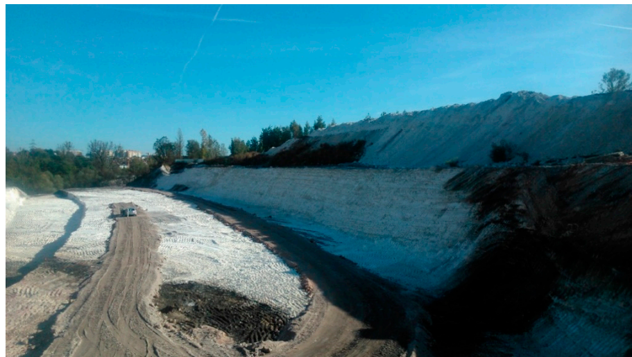
Figure 2. Excavation during the construction of the Łagiewnicka route in the “White Seas” area (photo Pilecka).
