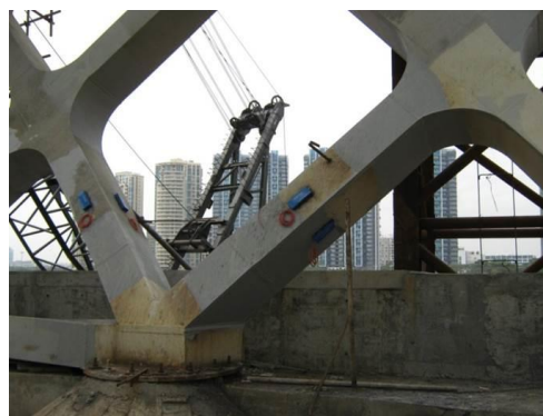
Figure 3. The sensor installation of two support connecting rods.
