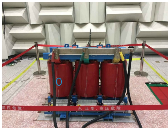
Figure 35. The transformer in the field test.
