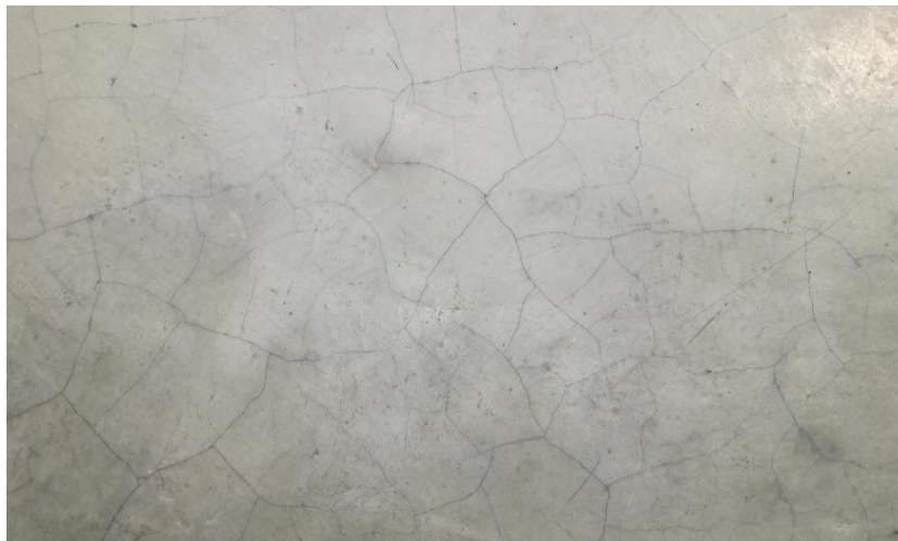
Figure 5. Early-age map cracks that occurred in a newly cast concrete floor slab; these cracks appeared within 14 days of concrete placement; the floor slab was cured by spraying of water.
