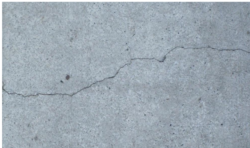
Figure 6. Restrained shrinkage cracking that occurred in a roadside concrete curb; this crack initiated within 56 days of concrete placement; the curb was cured with curing compound.
