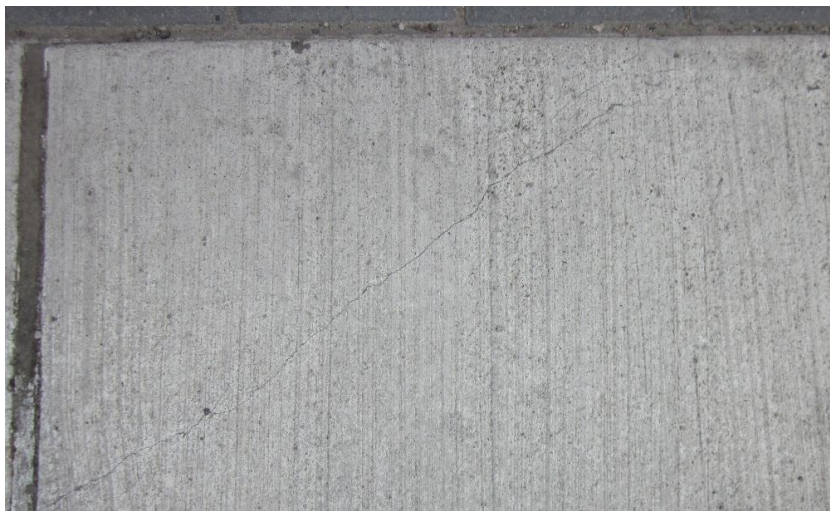
Figure 3. Early-age corner crack in a concrete side-walk slab; this crack appeared within 35 days after concrete placement; the concrete slab was cured by curing compound.
