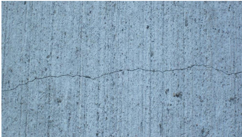
Figure 2. Early-age transverse crack in a concrete pavement slab which widened over time; this crack started within 56 days of concrete placement; the slab was cured using curing compound.
