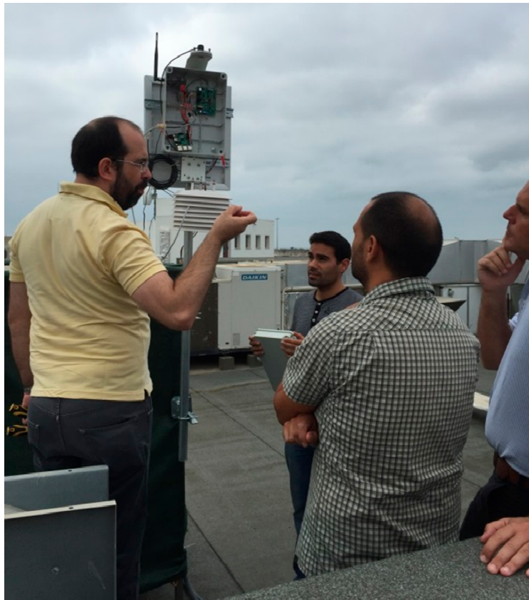
Figure 25. Installation of the intelligent weather station.
