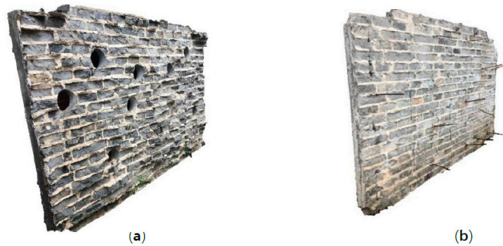
Figure 14. The interface between the strengthening layers and the masonry substrate: (a) The coarse interface between the UHPC layer and the masonry substrate; (b) The smooth interface between the reinforced polymer mortar layer and the masonry substrate.
