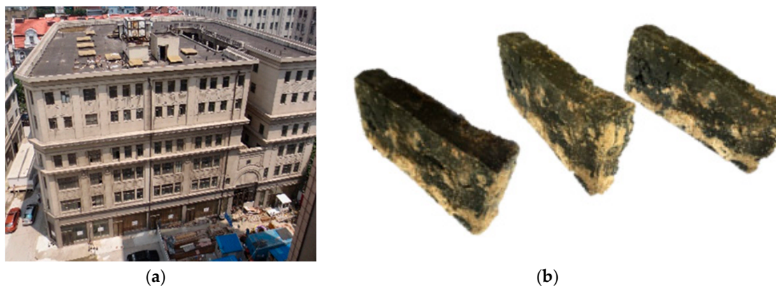
Figure 1. The historical building and bricks: (a) The historical building under rehabilitation; (b) the bricks sampled from the historical building.
