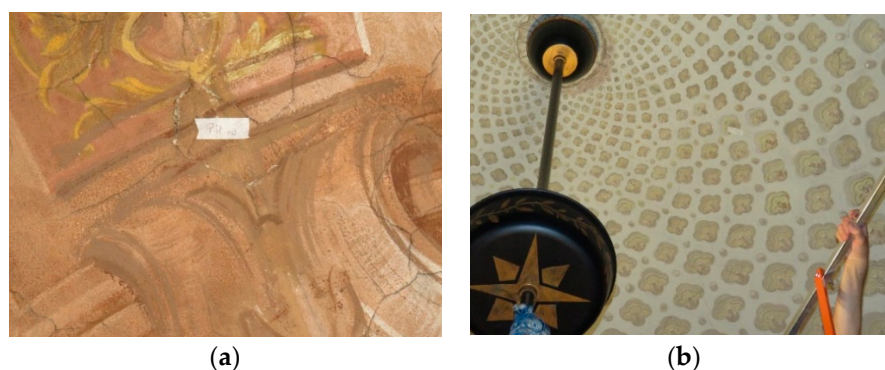
Figure 14. Points of potential plaster detachment: (a) P11 vault Pelagi room; (b) P15 vault Giunta room.
