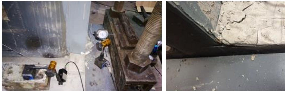
(a) buckling of side plates and pulling failure of weld joints
