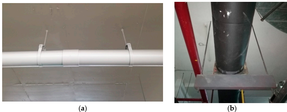
Figure 1. Two types of suspended piping systems: (a) A single rod piping system; (b) trapeze hangers supporting a suspended piping system.
