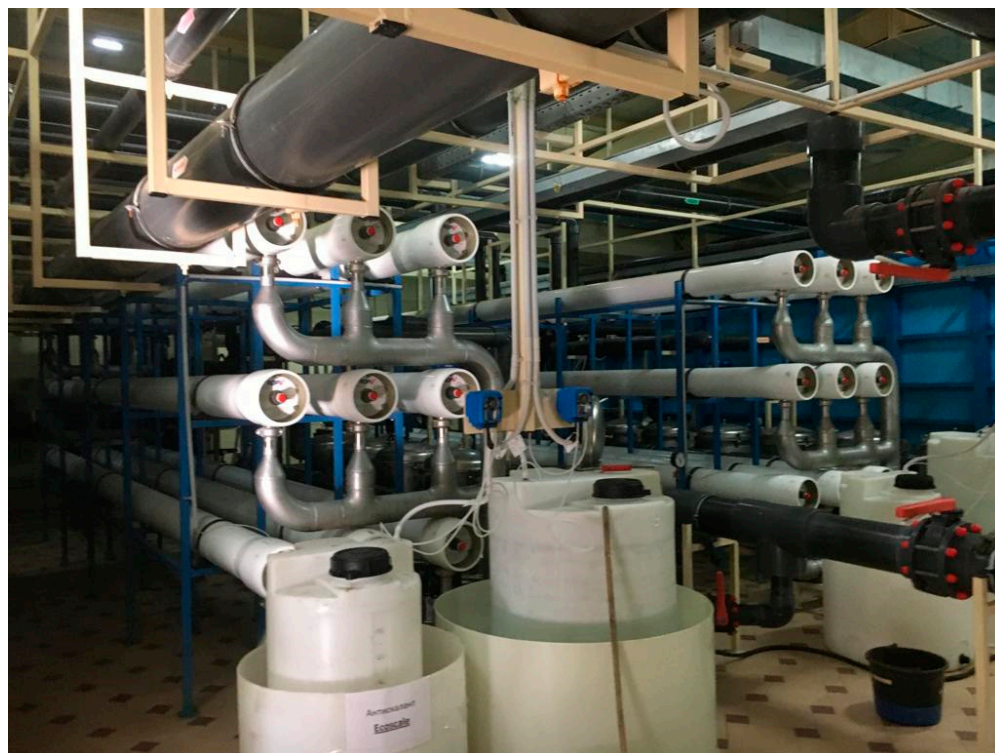
Figure 8. A 120 cubic meter per hour reverse osmosis membrane plant for production of drinking quality water from the ground water well intake in the Moscow region.
