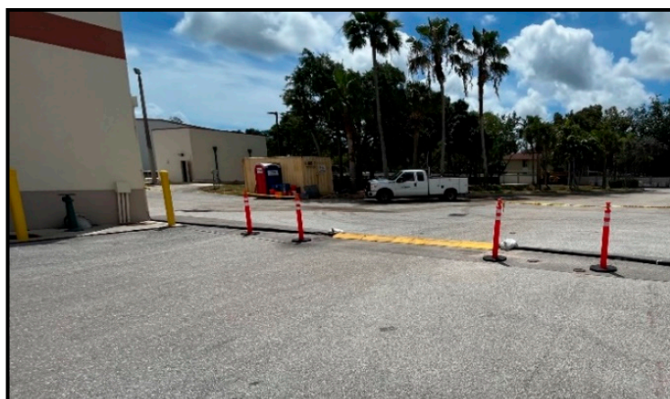
Figure 3. NF concentrate transfer pipeline between NF and RO process rooms.
