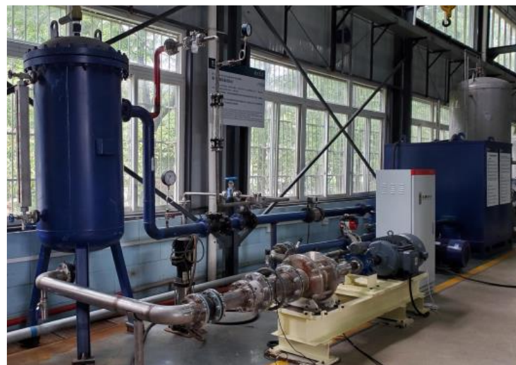
Figure 5. The multiphase pump test system.
