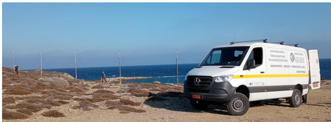
Figure 13. Installation of the linear receiver array of the “Dardanos” system in the Plaka site (north-eastern extremity of Lemnos Island) in December 2020.
