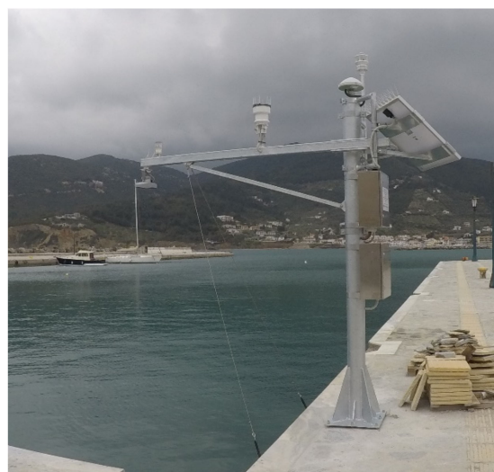
Figure 11. A radar tide gauge equipped with meteorological sensors and wireless telecommunication link, installed at Skopelos Island.
