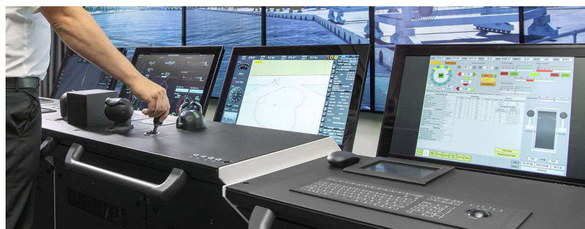
Figure 5. ABB Ability™ Marine Pilot Control system [15].
