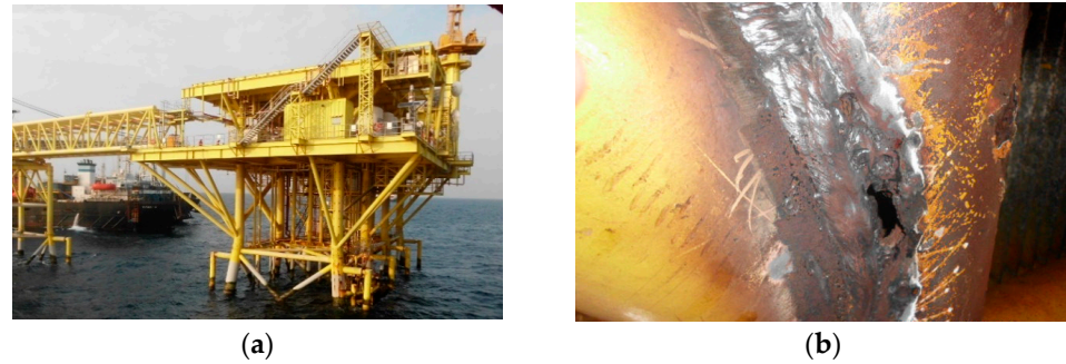
Figure 1. Drilling platform (a) profile view and (b) joint damage.
