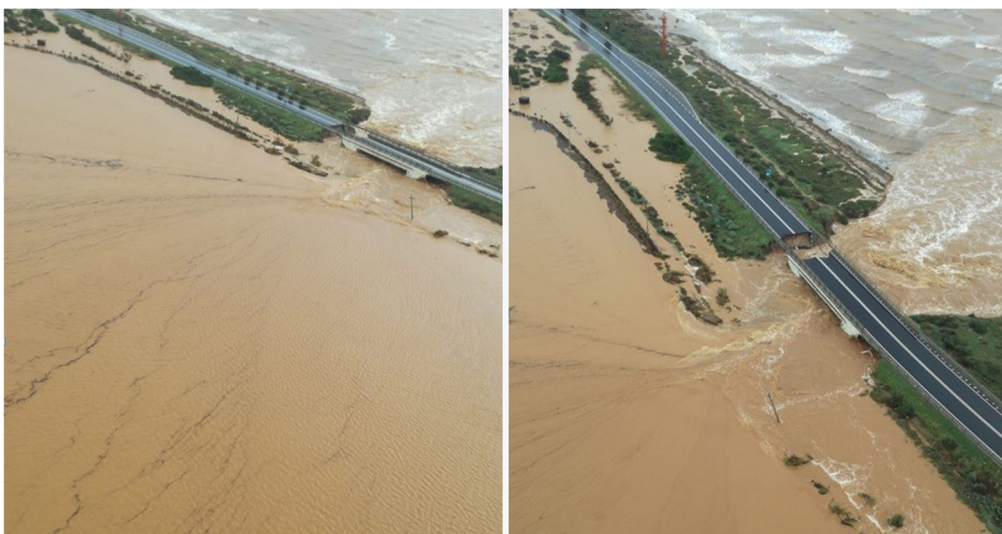
Figure 5. Barrier breaching at La Playa beach and collapse of SS 195 during the compound sea and lagoon flood of 10 October 2018.
