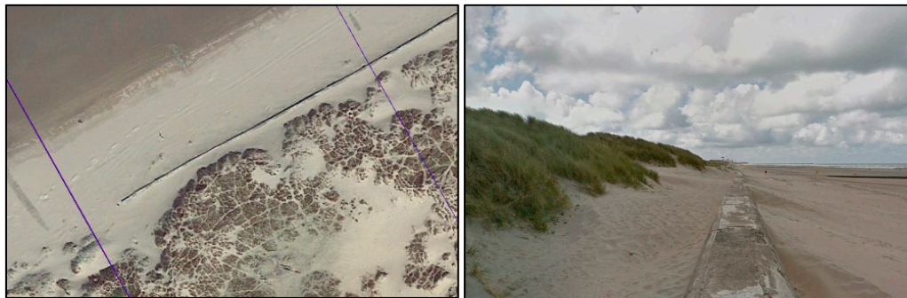
Figure 17. Concrete wall as a dune foot protection measure in section 72.
