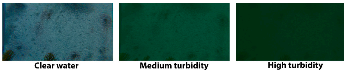
Figure 13. Image of a corroded surface on a wharf captured under clear, medium turbidity, and high turbidity conditions.
