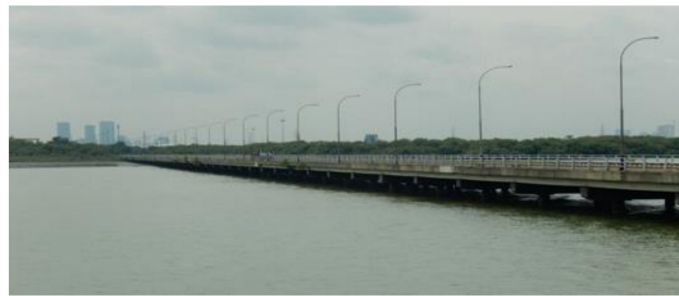
Figure 1. The view of the RC bridge in TPS (from the domestic harbor).
