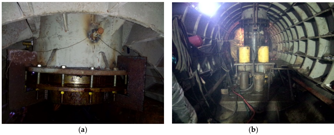
Figure 2. Construction process of the VTM: (a) The embedded first standpipe section; (b) Construction diagram on site.
