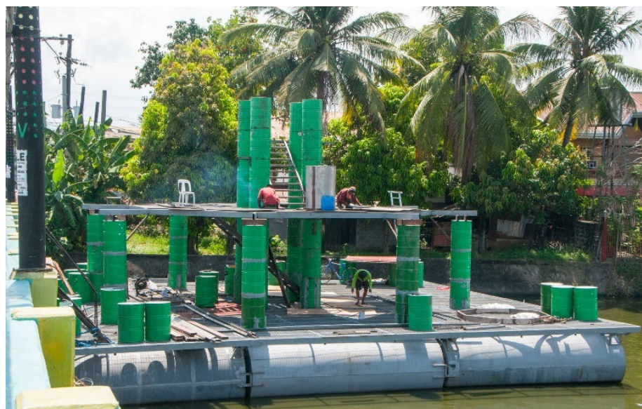
Figure 8. The building process of the pagoda. Note: Courtesy of Engr. Rodelio Mendoza Concepcion; permission has been given to the authors for the publication and reprinting of this photograph.
