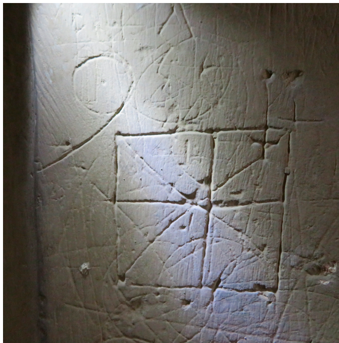
Figure 4. A portion of a pier in Stradishall that contains the majority of graffiti in the church. It can be observed there is a wide variety of inscriptions overlapping in a palimpsest.
