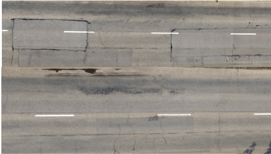
Figure 9. Cropped sections of the pavement model's surface (( top ) image shows a cracked and rutted sub-section and the ( bottom ) image shows a sub-section with depression, cracking and rutting distresses).
