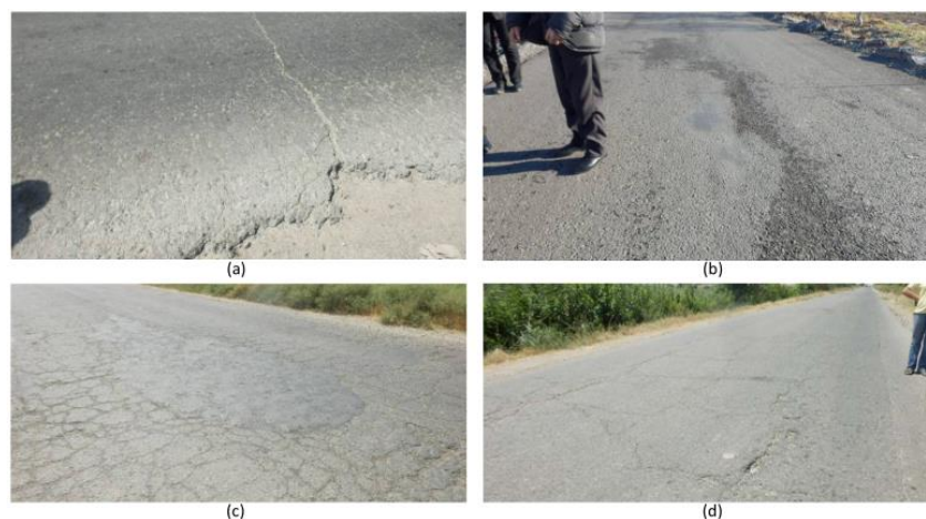
Figure 2. Examples of the percentage of cracks [18] are (a) new pavement, 0% cracks; (b) partial cracks, 1–50%; (c) partially connected cracks, 50–70%; and (d) dense and mixed cracks, 70–100%.
