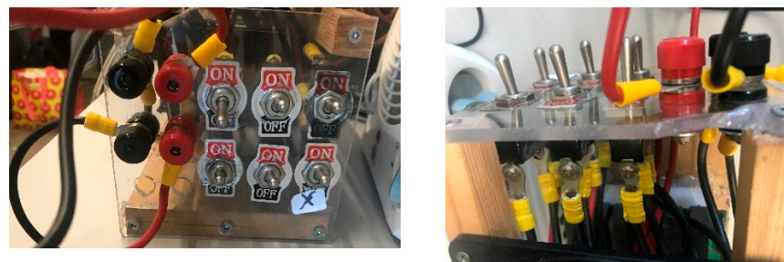
Figure 4. Image of the switch set that controls the capacitor bank.
