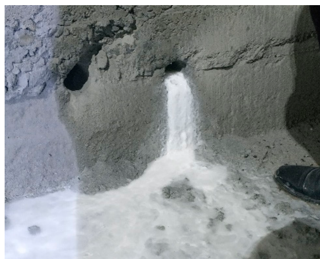
Figure 1. Crystallization and clogging in drainage pipes in the Baoligang Tunnel of the Emeishan-Hanyuan Expressway.
