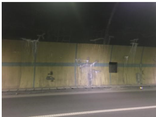
Figure 2. Cracking and leakage of the tunnel lining.
