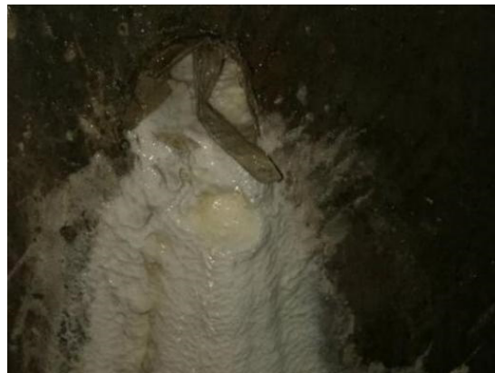
Figure 1. Blockage of a tunnel drainage pipe caused by crystals.
