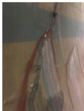
Figure 2. Cracking of the tunnel lining.
