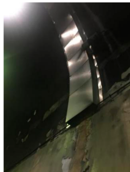
Figure 1. Water receiver at lining leakage.
