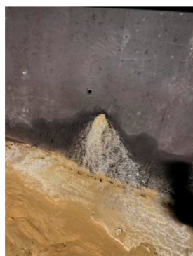
Figure 3. Tunnel drainage pipe blockage by crystals.
