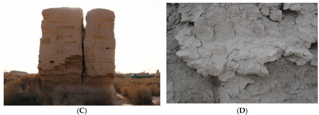
Figure 2. The deterioration of earthen sites in China. (A) Collapse; (B) sapping; (C) cracks; (D) weathering.
