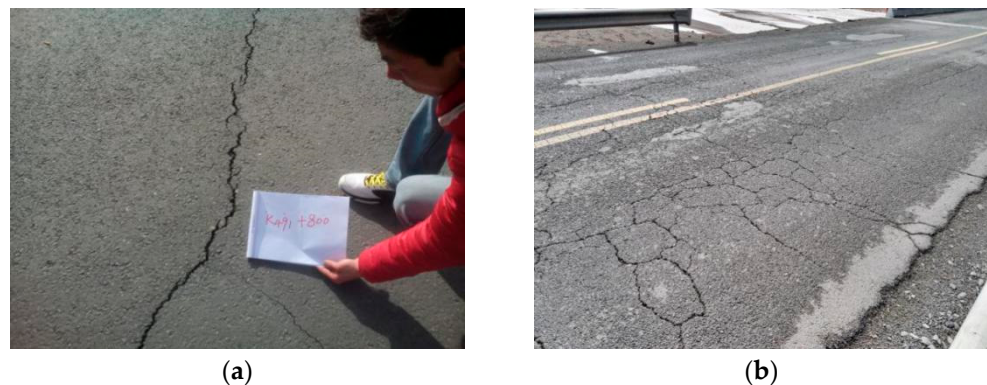
Figure 3. Lateral cracking and network cracking problems of asphalt pavement. (a) is transverse crack; (b) is net crack.
