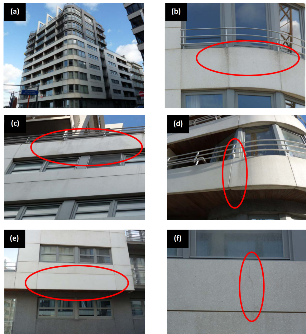
Figure 4. Residentie Commodore (Ostend, Belgium), the first Belgian self-cleaning building which evidenced low photocatalytic performance after 4 years of construction [34]. (a–c) facade, balconies and walls evidenced dirty surfaces (d,e) balconies and walls evidenced different white intensities, (f) cracked surfaces.
