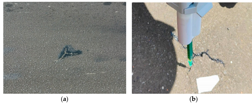
Figure 8. Irregular cracks on XHMB pavement. (a) chicken-feet crack, (b) irregular crack.
