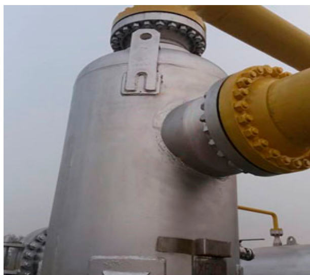
Figure 1. A large cyclone separator in a natural gas station.
