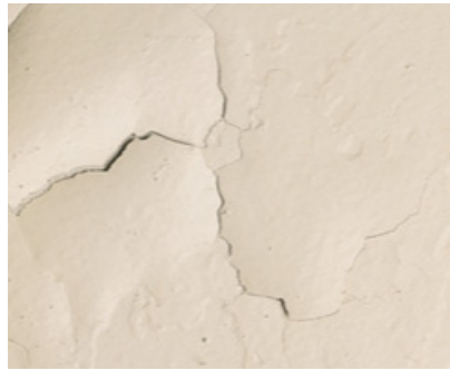
Figure 6. Cracking, bubbling and loss of paint adhesion to the substrate caused by high levels of moisture [1].
