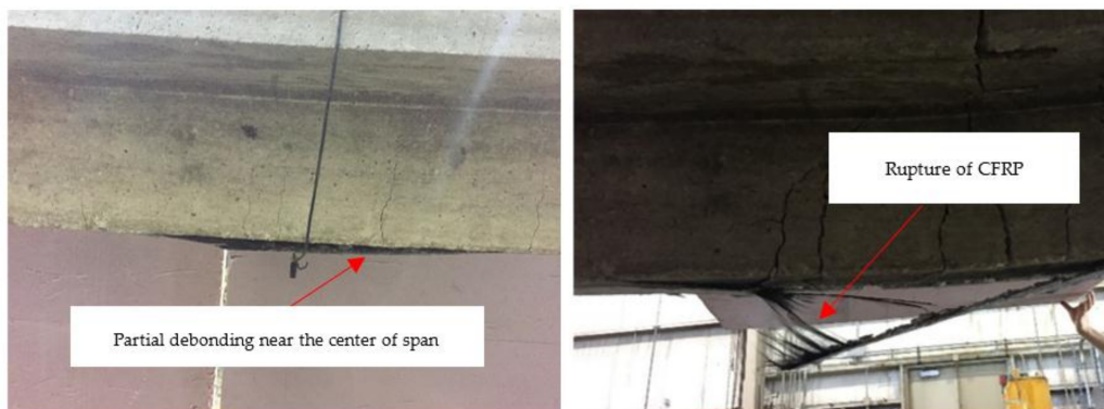
Figure 10. Typical debonding (Left) and rupture (Right) of beams (B2–B4).
