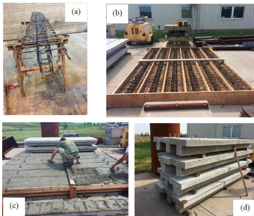
Figure 3. Casting of the T-beams: (a) steel reinforcing cage, (b) formwork with the reinforcement cage, (c) T-beams during casting, (d) T-beams removed from their formwork.
