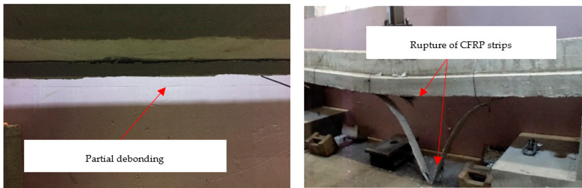
Figure 17. Typical debonding (Left) and rupture (Right) of beams (B14, B15, and B17).
