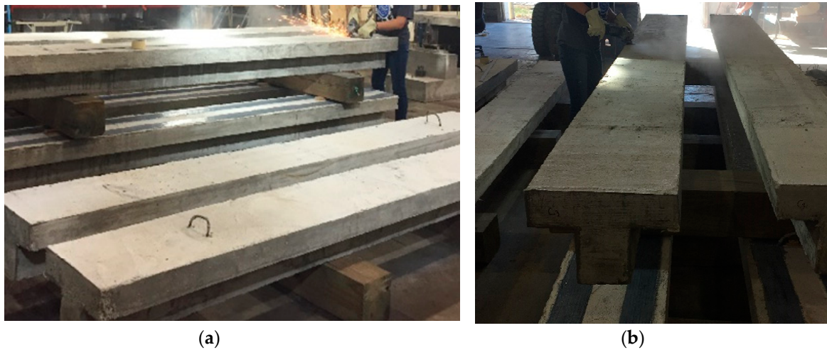
Figure 5. Surface preparation: (a) the inverted T-beam before lifting hooks were removed; (b) concrete surface grinding.
