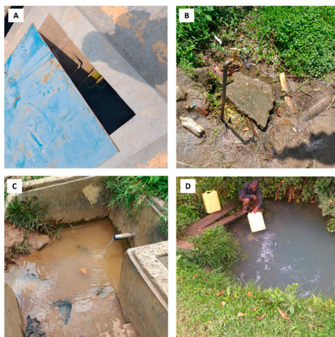
Figure 2. Photos of observable risks to water infrastructure in the study area: (A) a reservoir containing algae growth (greenish color on the inside stairs); (B) a tap stand with poor drainage; (C) a spring with an outlet pipe and inadequate drainage; and (D) an unprotected spring.
