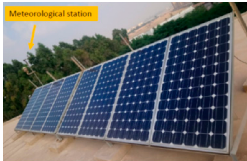
Figure 1. Monocrystalline photovoltaic system on the roof of Heliopolis University.
