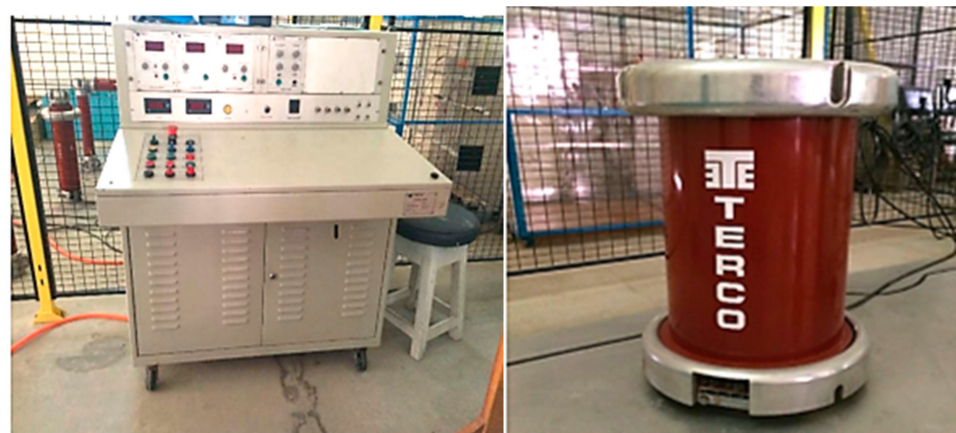
Figure 6. Control desk and test transformer.
