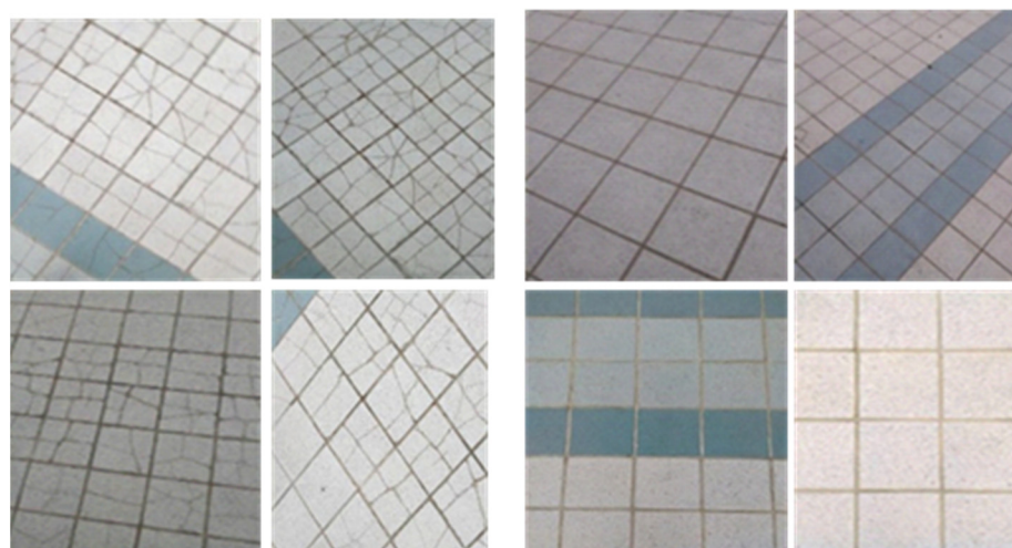
Figure 5. Left, Tile Sample with Crack; Right, Tile Sample without Crack.
